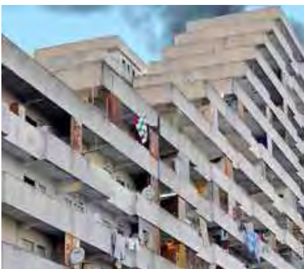
The Vele di Scampia, Sails of Scampia, constructed 1962 – 1975. Today in a state of decay, although still occupied by residents.
